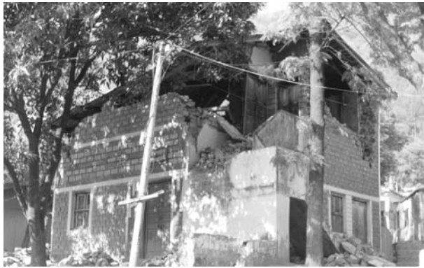
Figure 7.1 : A Damaged Building Due to an Earthquake
